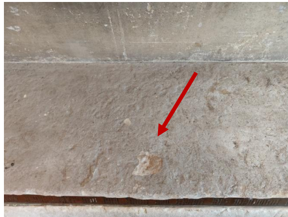
Figure 31 show the paint flaking in the central area of the stone seat.
