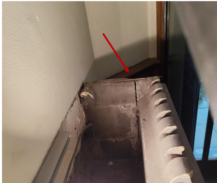
Figure 29 show the iron supporting the crenelation.
