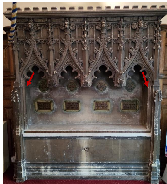
Figure 30 show the point where metal was detected, likely iron dowels.
