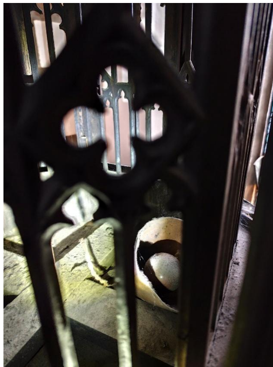
Figure 17 redundant light system internally.
