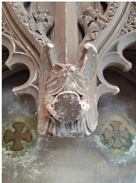
Figure 35 show the iron dowel used to support the angel head with active oxidation.
