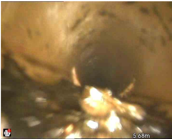
HOLX_de0a0591-9f40-4000-95a9-1d120054087b_20241204_094912_845.jpg, 00:00:25, 6.00 m Joint displaced, large
