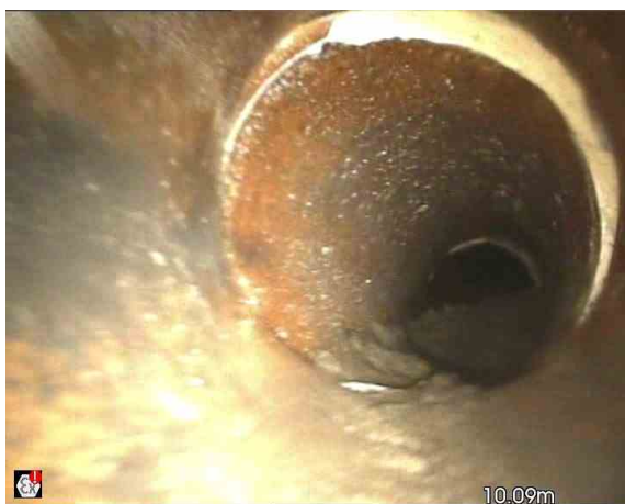
HOLX_b332ada4-07d8-4aa5-a926-19bf2996e49c_20241204_115919_896.jpg, 00:00:33, 10.30 m Joint displaced, large
