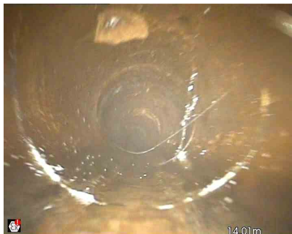
MH5X_175cf094-4b0a-4ec2-a684-b70b6543e0f9_20241204_111100_422.jpg, 00:01:18, 14.30 m Hole in drain or sewer at 11 o'clock
