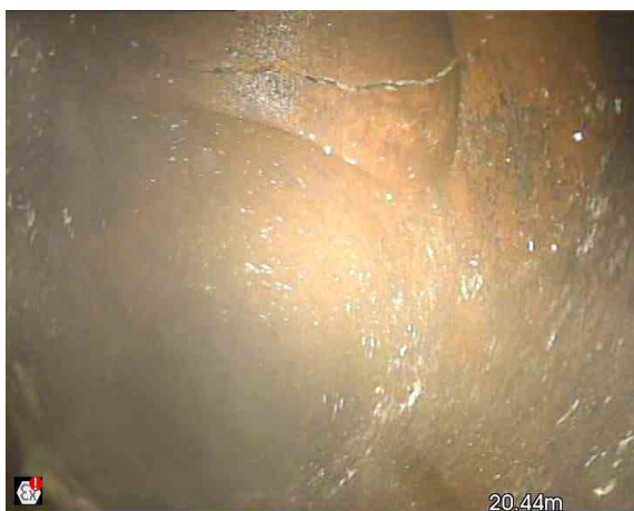
MH5X_abe27e89-56a8-431a-99ec-3d3ba66a8485_20241204_111530_717.jpg, 00:01:44, 20.60 m Fracture, circumferential from 10 o'clock to 2 o'clock, inside connection
