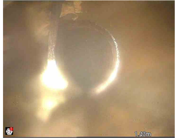
MH5X_c0c3a63c-6cdc-4a35-a548-ab103acfaab9_20241204_101307_004.jpg, 00:00:08, 1.80 m Other obstacles from 7 o'clock to 11 o'clock, 10% cross-sectional area loss, through pipe wall
