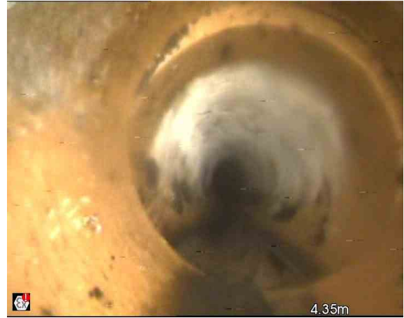
HOLX_8fe7d4a0-a447-4f32-8652-4e34f0c8edb9_20241204_094802_729.jpg, 00:00:22, 4.50 m Joint displaced, large
