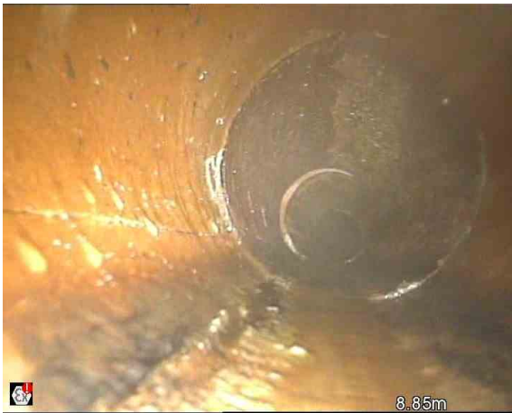
MH5X_185be66f-17c8-4d9e-bd18-b977a3fbfb20_20241204_101449_021.jpg, 00:00:52, 8.70 m Crack, longitudinal at 8 o'clock, start
