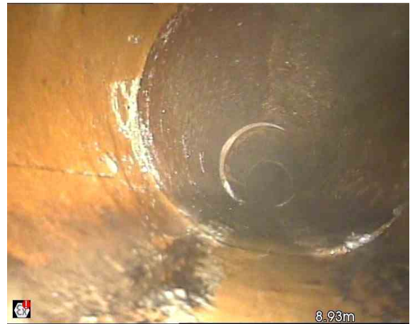
MH5X_6a26c413-ea11-457a-957f-f760f4e0470e_20241204_101453_766.jpg, 00:00:52, 8.70 m Crack, longitudinal at 8 o'clock, start
