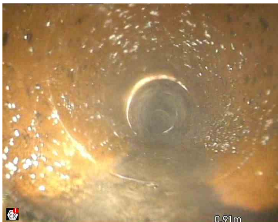
HOLX_b8521a0e-a45a-4bdd-8b27-920ac559ada8_20241204_115742_254.jpg, 00:00:11, 1.00 m Crack, circumferential from 12 o'clock to 12 o'clock
