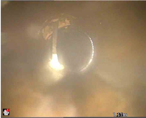
MH5X_9fc6e4c7-2a43-4a5b-87c7-f4a1d26bb878_20241204_101328_412.jpg, 00:00:07, 1.80 m Broken pipe from 10 o'clock to 12 o'clock
