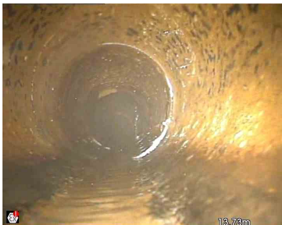
MH5X_d408e408-6f02-4475-9b5c-a995a6e660a8_20241204_111046_661.jpg, 00:01:17, 14.00 m Crack, circumferential from 7 o'clock to 3 o'clock
