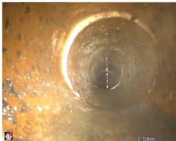
HOLX_8403c2cd-9572-4d5d-a5bb-ef0710bb80ff_20241204_115838_850.jpg, 00:00:12, 1.80 m Joint displaced, medium
