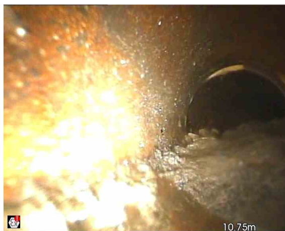
HOLX_6fb0ee1b-c051-431e-b61d-a9be6db5d8c1_20241204_115941_937.jpg, 00:00:35, 10.90 m Settled deposits, coarse, 40% cross-sectional area loss, start
