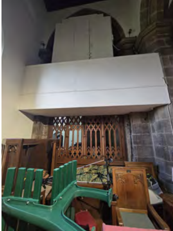
175. G9 Ground Floor South Wall South | No Scale
