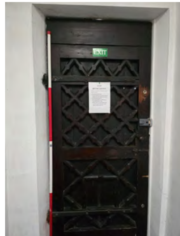
210. G13 South Wall Door Detail South | 1x2
